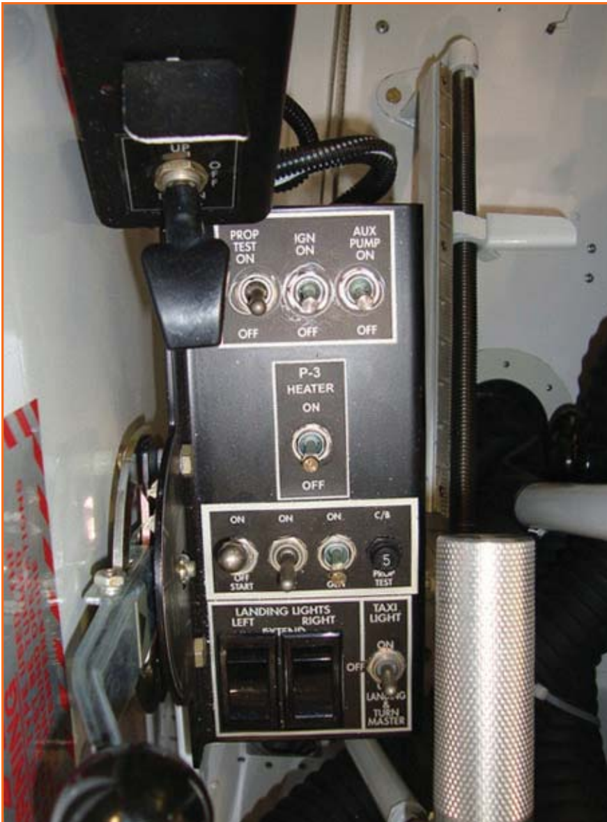
This is an example of the cockpit panel in a PT6-powered Turbo Thrush. The start switch is located in a small panel on the lower left side of the cockpit behind the throttle quadrant. It is on the aft part of the panel, next to the battery and generator switches, and the ignition switch is on the forward part of the panel.
