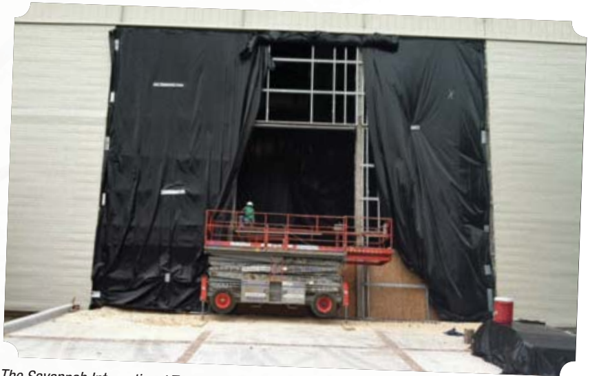
The Savannah International Trade & Convention Center installed hangar doors earlier this year to accommodate NAAA and its aircraft exhibitors. Thanks to this significant facility improvement, 10 airplanes and three helicopters will be on the trade show floor, including the recently FAA-certified Thrush 510G, the Thrush 510P, AT-502B, 602 and 802 Air Tractors, and a new entry to the ag market, the PA-25 from Laviasa.
